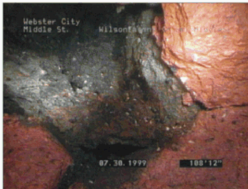
IMAGE: 11_4b, TAPE #: 1, 01:44:24 lateral broken at 09 o'clock
